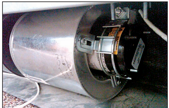
FIGURE 2. Retrofitted fan with ECM motor.
